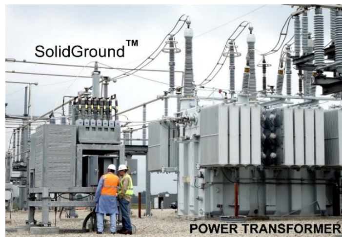
Figure2. SolidGround™ [4] by ABB (left) meant for blocking GIC in a neutral conductor of power transformer (right)
