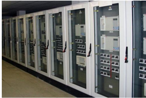
Figure4. Contemporary way of electronic equipment mounting in cabinets.
